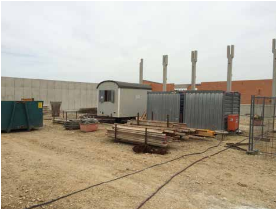
Fig. 4.1: Construction site of the sports hall “Am Sportpark, Zorneding” | Photo: Natalie Essig
