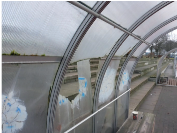
Defective walls of a shelter generally have sharp edges which can injure users.
