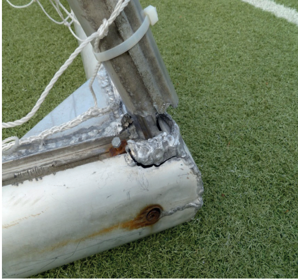
Backstay rewelded with the ground bar which with later use has split next to the welding seam.
