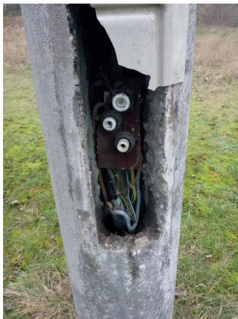
Publicly accessible electrical equipment. Interference by children can have serious consequences.
