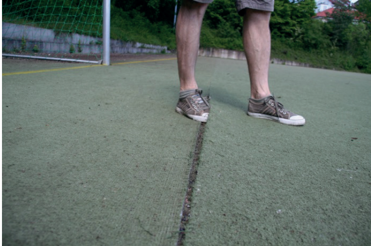
Open seams in synthetic grass surface. The surface is also very worn.
