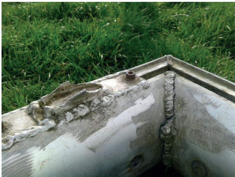
Rewelded bar that was later removed. Potential risk of injury from sharp edges.
