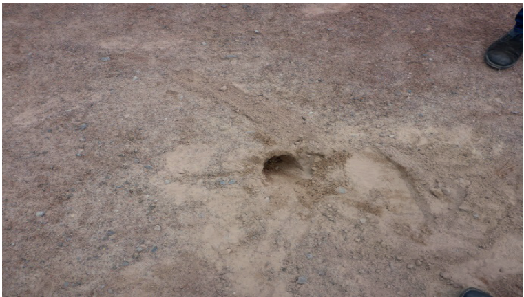
Holes in tamped surface and coarse grain on the covering layer
