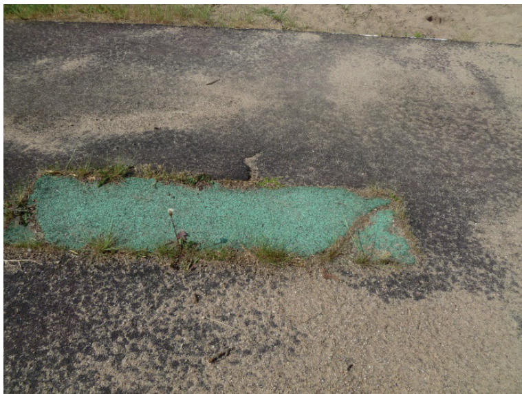
Defective surface and take-off board at the landing pit may cause users to trip and fall.
