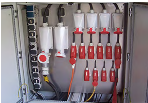
Stromanschlüsse TV Compound
